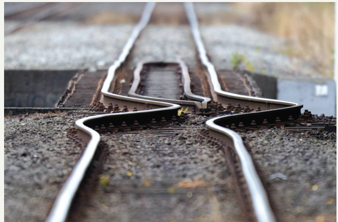
A rail line buckled by the shifting earth is pictured in Christchurch, New Zealand, on Feb. 23, 2011, a day after a deadly 6.3-magnitude earthquake rocked the city. Hundreds of rescuers swarmed twisted and smoking buildings in a frantic search for survivors. The catastrophic quake left nearly 400 dead or missing. ▶▶
