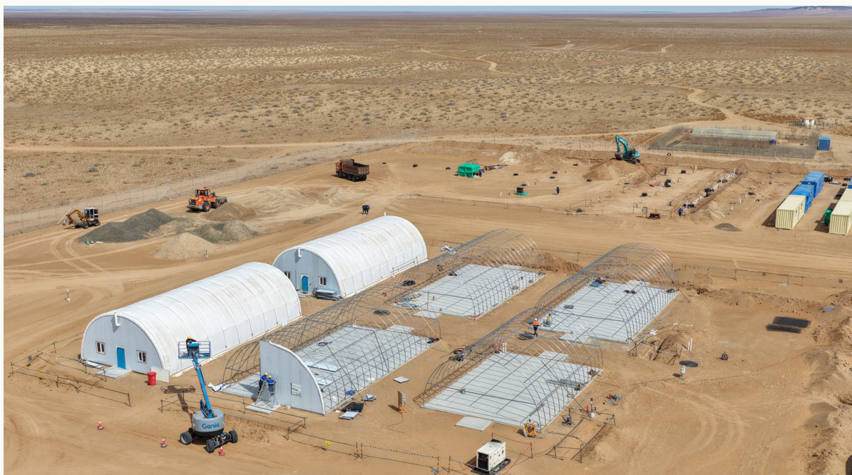
Construction of temporary facilities for the Zuuvch-Ovoo Project. Ulaanbadrakh soum, Dornogobi province
