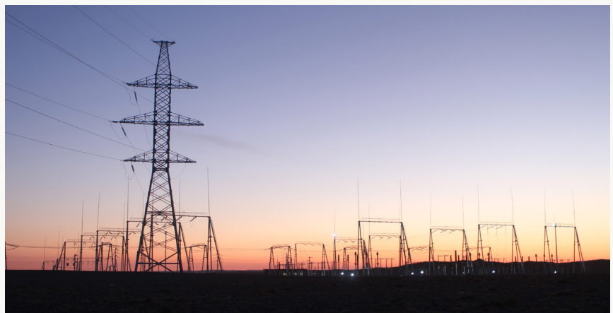
Nationwide electricity accessibility is at 90 percent
